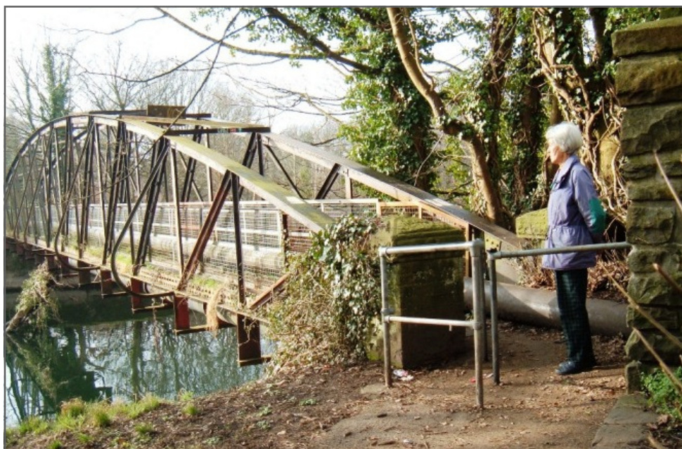
The pipe bridge at Clydach which the Connect2 route will bypass. Note the barrier in the foreground over which a bike must be lifted.
